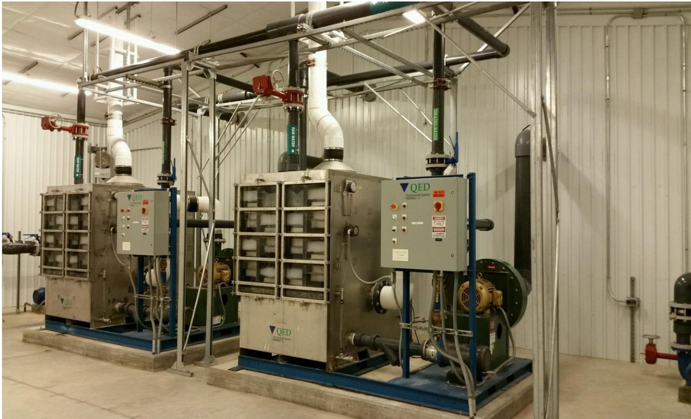
STACKED-TRAY AIR STRIPPER WATER TREATMENT SYSTEM
